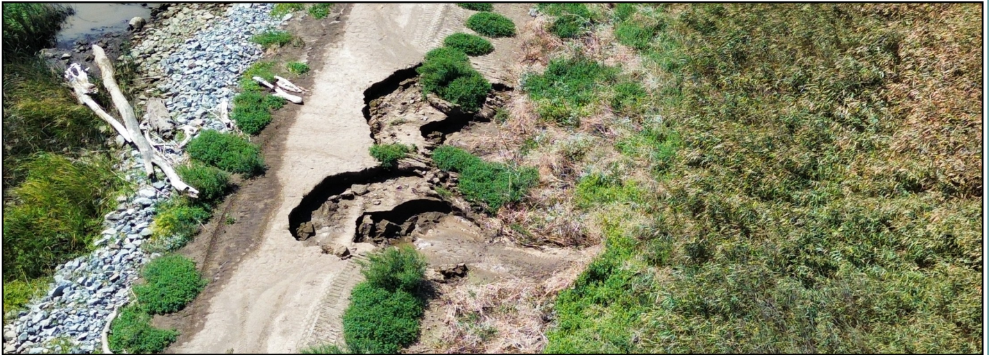
Higher-than-normal summer tides caused erosion from overtopping, as seen on this Suisun Marsh levee.
