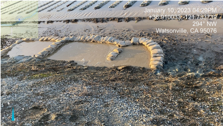
U-Shaped Sack Ring (looking from the levee crown towards the landside toe)
